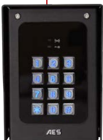
Gate/Entrance 4 Auxiliary Prox & Keypad Unit
